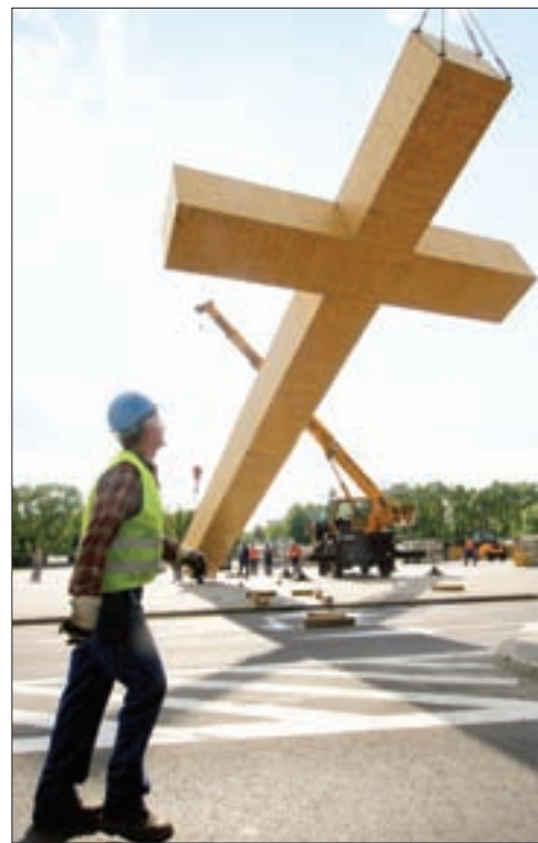
Workers erect a wooden cross on the altar that will be used for Pope Benedict XVI's Mass in Warsaw (Photo: CNS)
